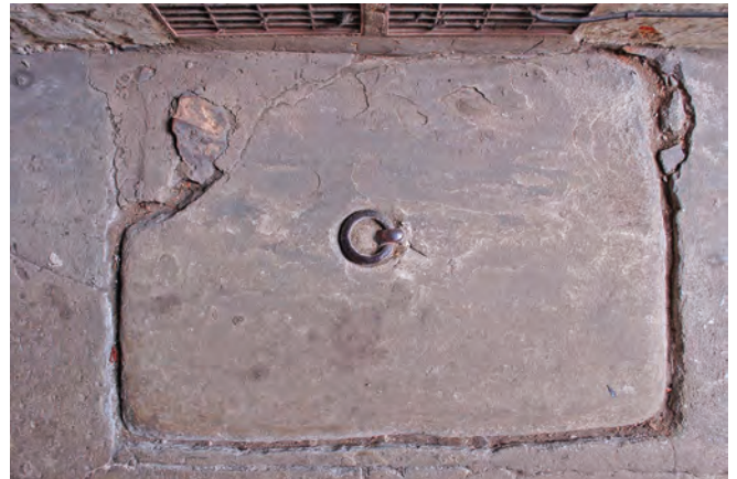
Coal/log chute seen from above. A similar hand-carved, ringed stone cover also serves number 12, next door
